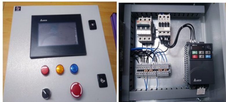
Fig: 5.8.3 (b). Consultancy Project: VFD and HMI Drive Panel using MODBUS protocol
